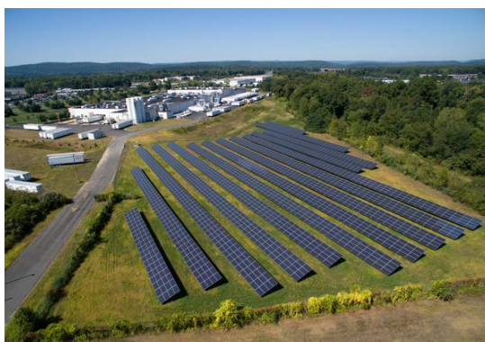
Figure 9 . View of the solar PV plant at Pepperidge Farm (Credit: Pepperidge Farm)
